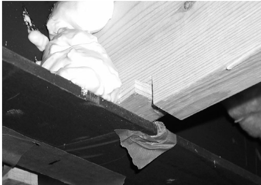
Figure 11-10. Photo showing method of temporary support for ceiling members and foam for permanent support.
