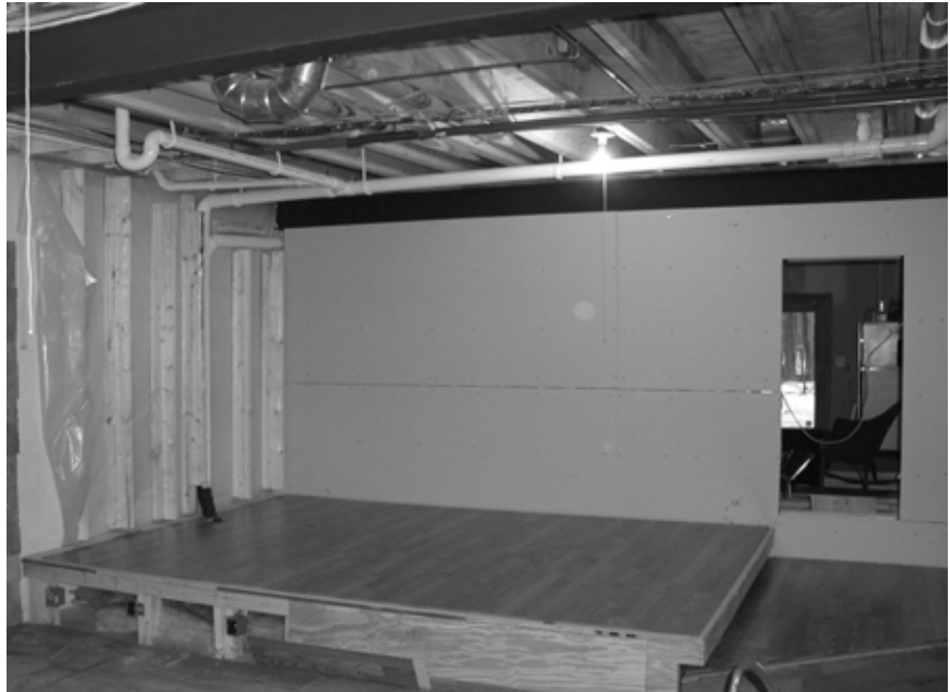
Figure 11-6. Photo of rear wall of HT under construction showing the opening for the equipment cabinet and the passive absorber riser structure.
