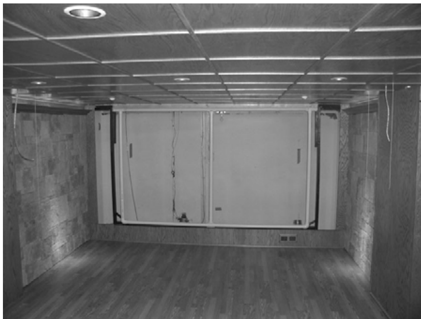
Figure 11-12. Completed room structure shown looking towards the screen area. Note the cultured stone on the two side walls and the frame for the screen made out of PVC. Also note the wood trim along the ceiling panels and the cove lighting at the side walls.
